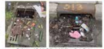
Garbage and Debris Collected At Storm Drain Grates
